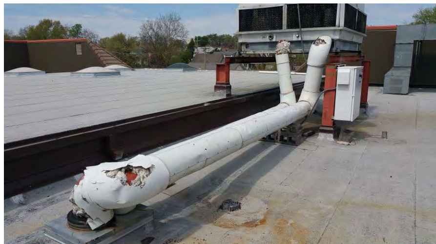
Existing Tower Piping
