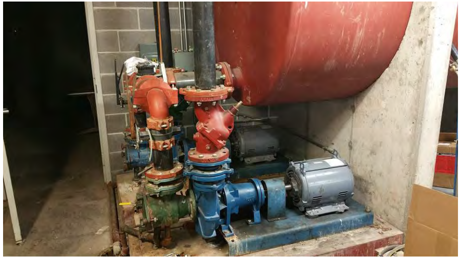
Existing Tower Pumps
